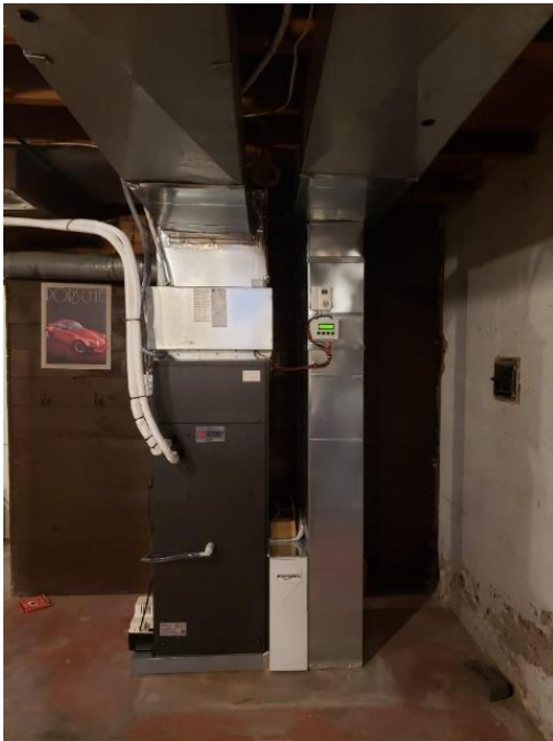
Figure 2 - Central Ducted ccASHPs appear similar to an oil furnace and use similar ducting to circulate hot air around the home.
