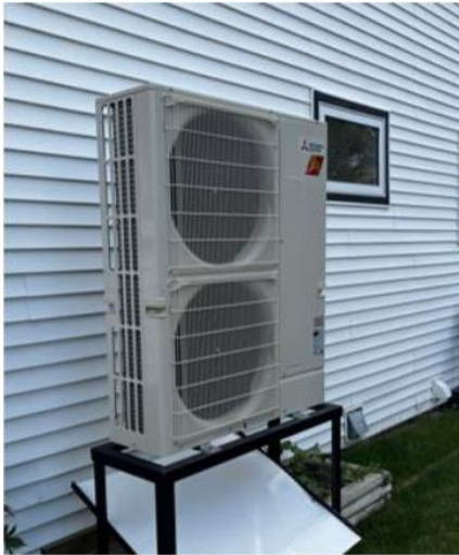
Figure 1 - Heat pump outdoor unit. This unit has been mounted well off the ground leaving room for ice buildup underneath. It is situated away from walkways, so ice removal is not needed. Outdoor units for ductless or central ducted systems are similar.
